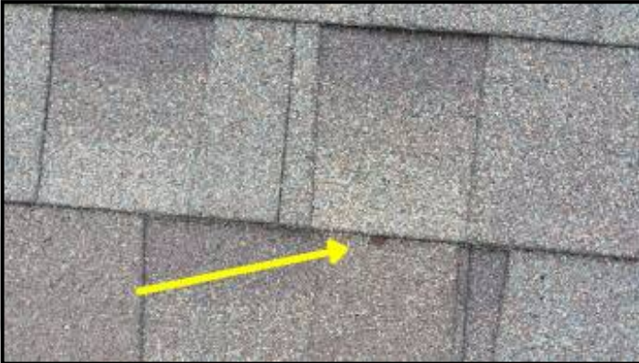
Exposed nail head on the south side of the roof.
