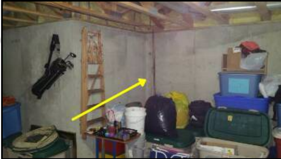
Main shutoff valve location.
