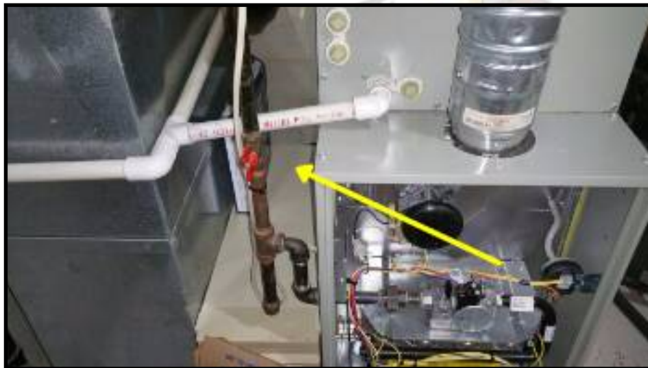
Furnace gas shutoff valve.
