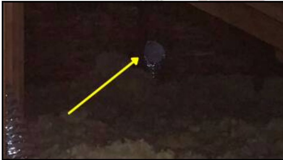
Attic Exhaust Vent
