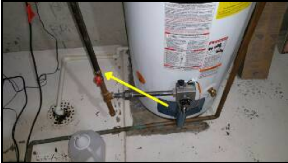
Water heater gas shutoff valve.
