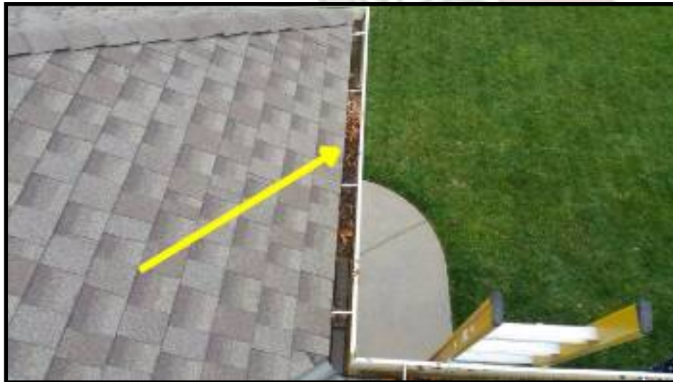
The gutters are clogged with debris.
