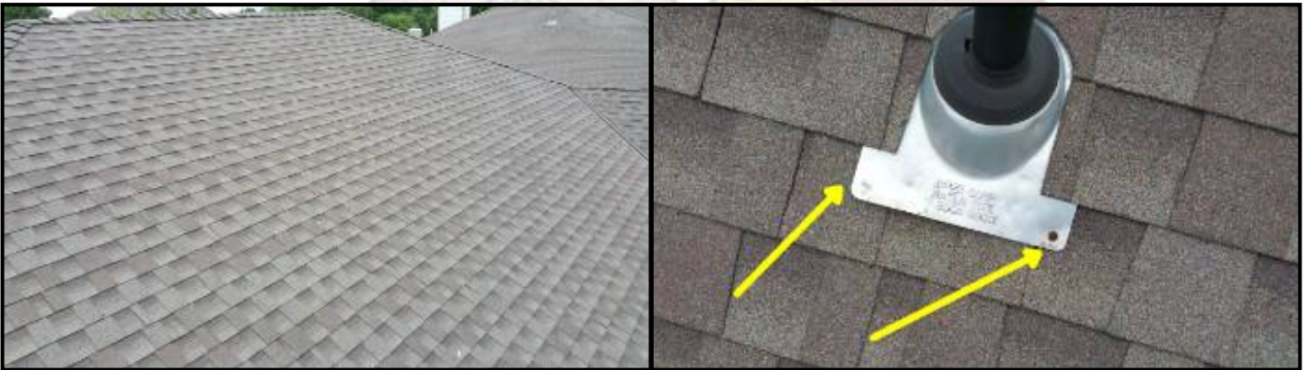
A nail is missing in the flashing and all others need to be sealed.
