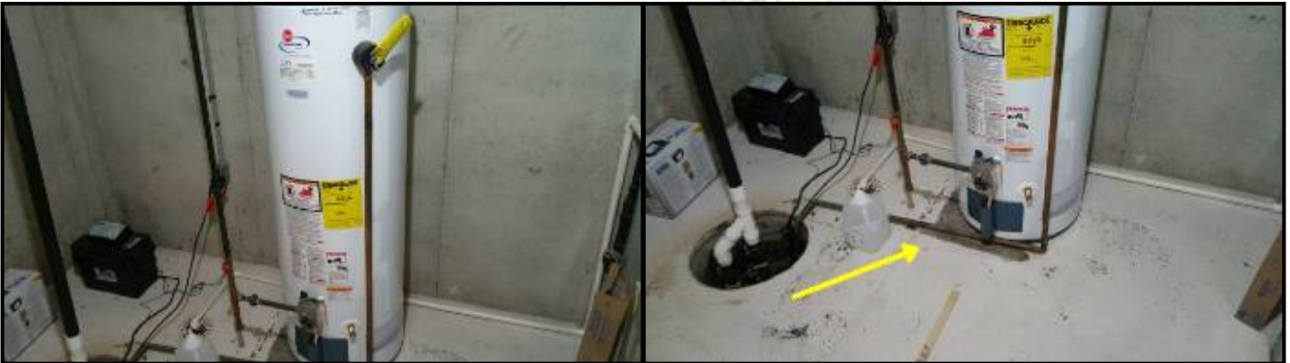
TPR valve draining into the sump pit.
