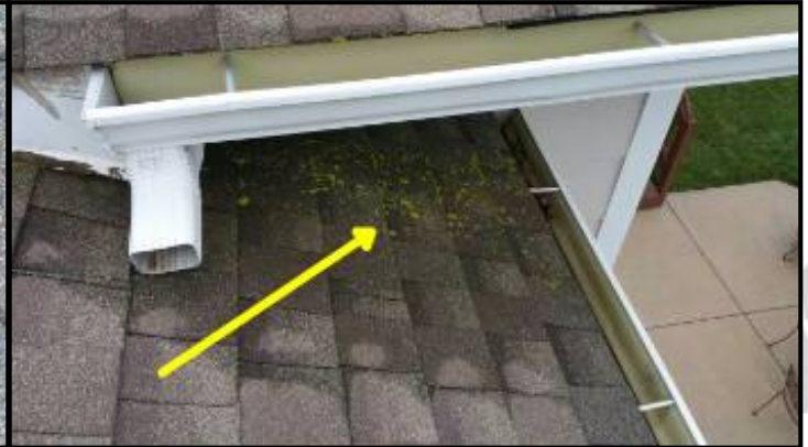
Moss growing on the roof
